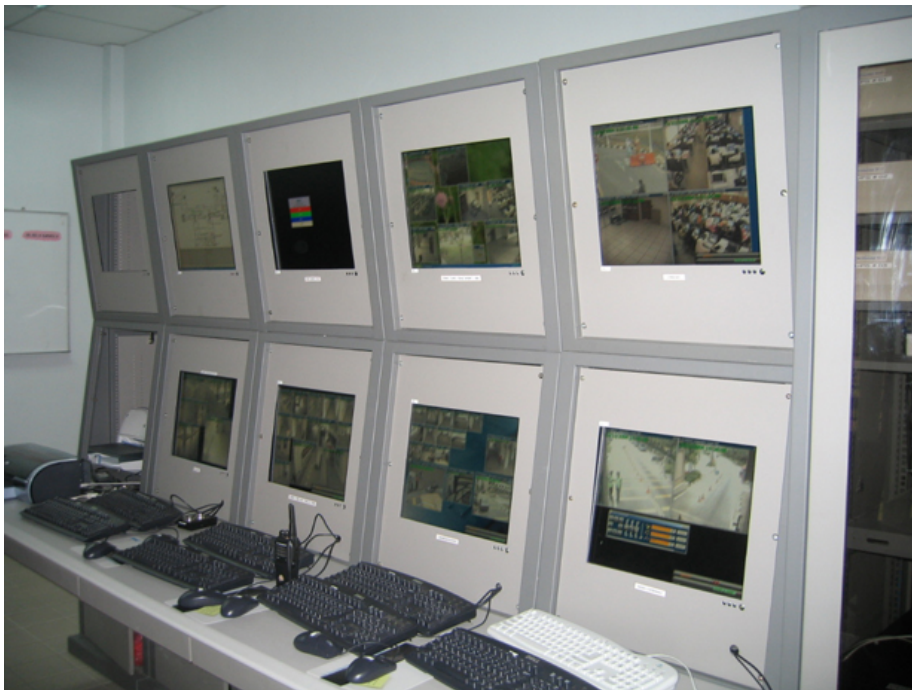
Figure 1: CCTV Control Panel Monitoring System
