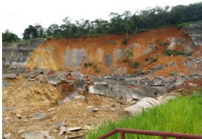
Figure 1.2: Photo on soil nailed wall failure at MRSM Bentong in 2009
