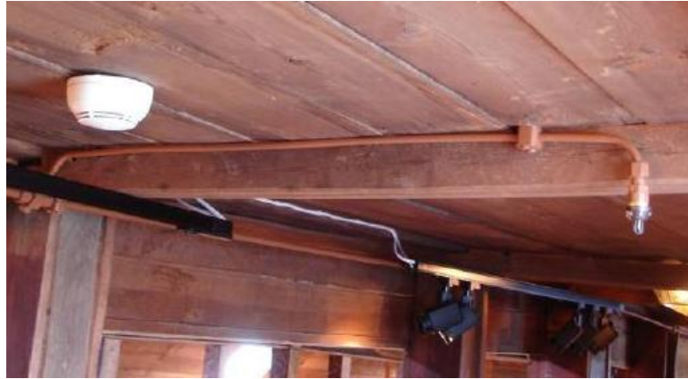
Figure 1.2: Exposed sprinkler piping and smoke detector (Source: Arvidson [2006] )
