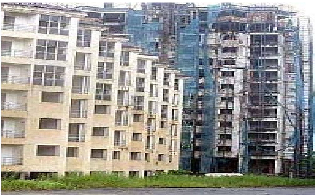
Figure 1.1: Condominium stands abandoned more than 10 years in Sentul- East Source: Field survey 2009
