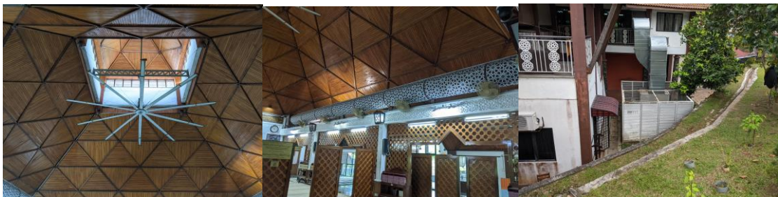
Figure 1.5 Giant Fan, Flex Ducted Air-condition system - source field survey
