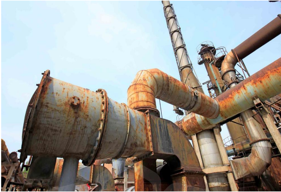
Figure 1.1 Corroded Industrial Boiler
