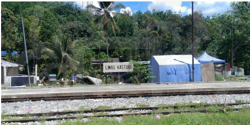
Figure 1.2 Train station building at Limau Kasturi, Gua Musang, Kelantan was damaged by flood happen in 2014
