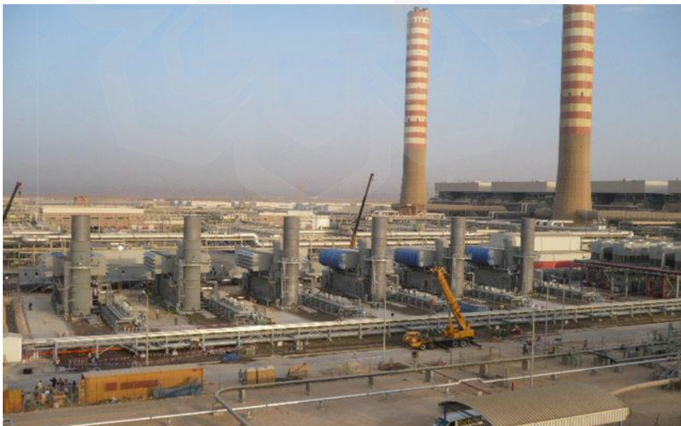
Figure 1. 2: Sabiyah Thermal Power Plant (CCGT Power Plant)
