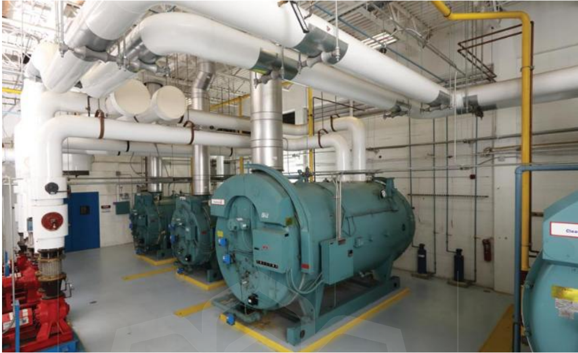
Figure 1.2 A series of the boilers with pipes used in it (Kleva, 2009)
